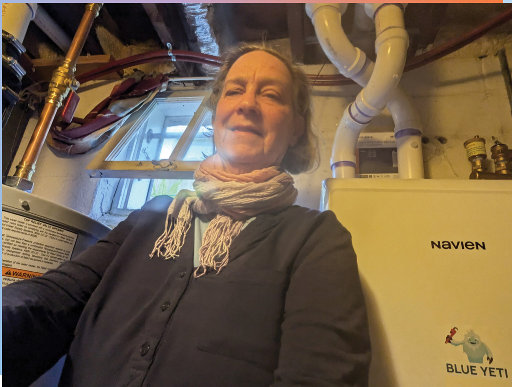
Sharee, Energy Assistance and Energy-Related Repair client, standing between her new boiler and water heater
